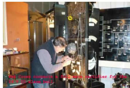
Pat Cross connects up a 24v rectifier for a DC Alarm Bell.
